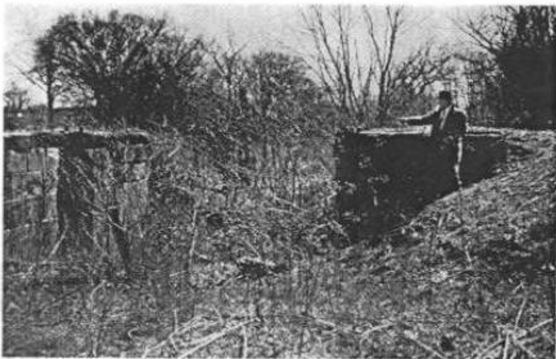
Shown here are the remains of "Four Mile Locks" at Fisher Bend south of Columbus. It is another project for restoration.
